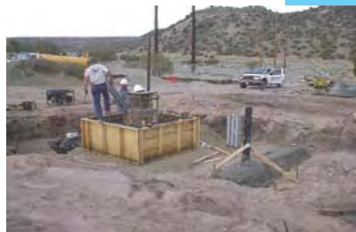
Crews work on a well under construction at the Buckman well field.
