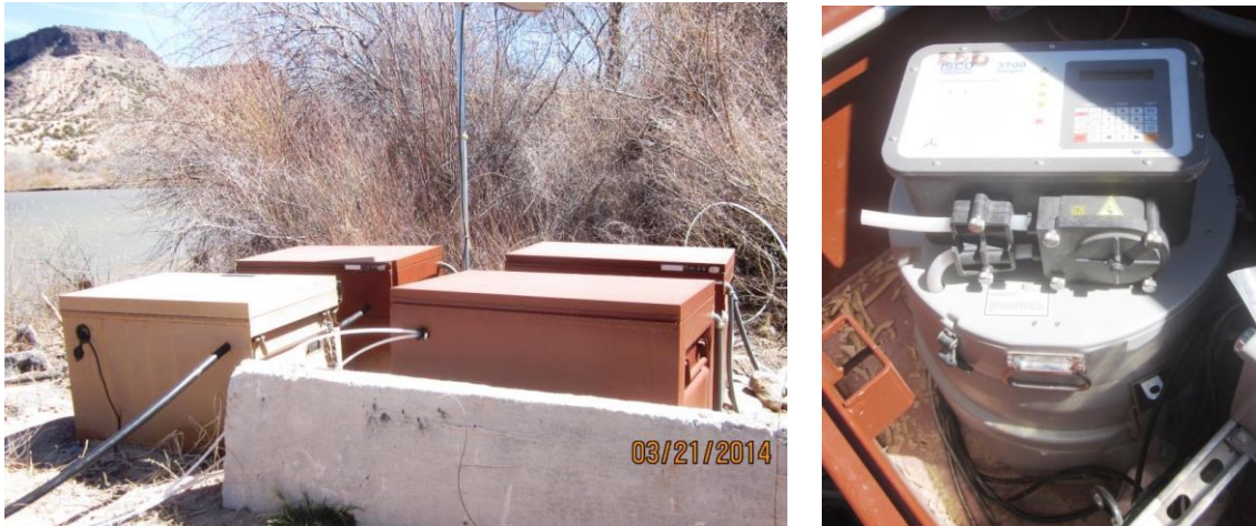
Figure 6. BDD intake station set up.
